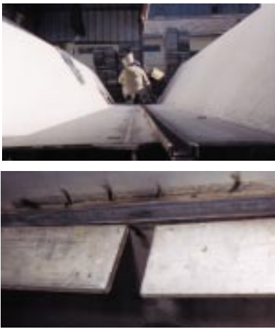
Figure 8: Welding of a corrugated bulkhead. Root (below) made with FCAW; filling and capping with SAW.
