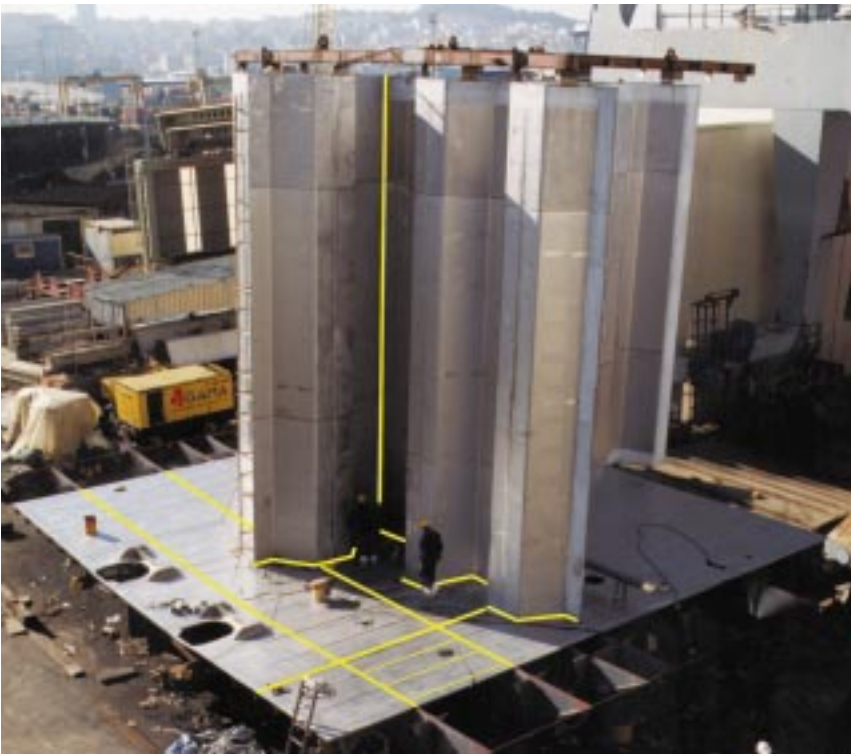
Figure 4: Fabrication of a block section consisting of a tank cover with vertical corrugated walls in duplex stainless steel.
