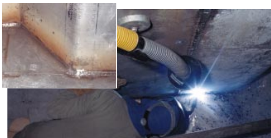
Figure 6: Attachment of a vertical corrugated tank wall to the tank floor; manually with OK Tubrod 14.27 (PC position).
